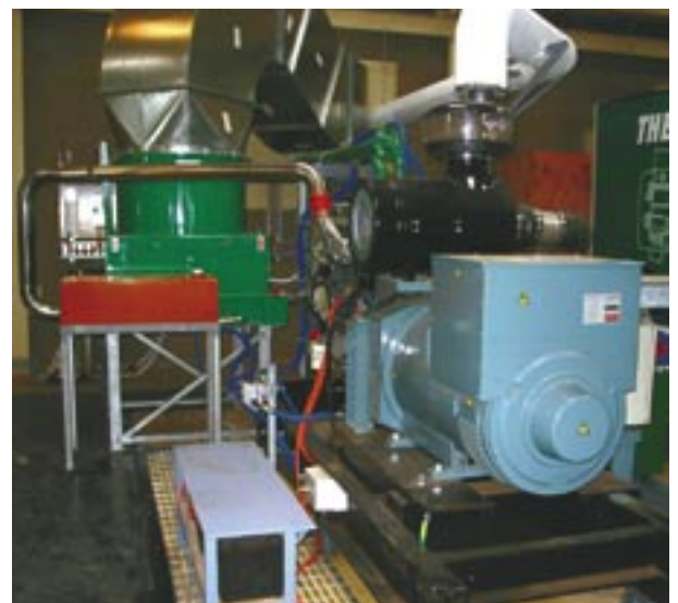
The Low Load Diesel in the Denham power station.
